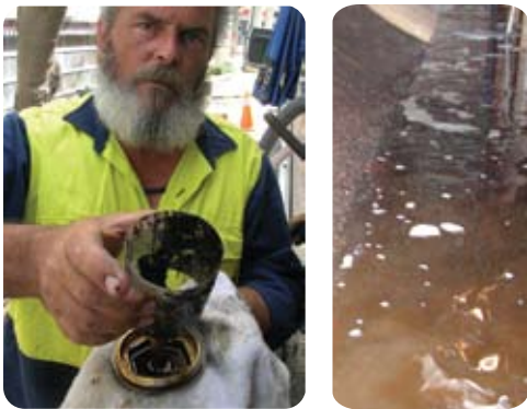
(Above) Left: A Leighton O'Brien field engineer holding a fuel tank filter that is covered in sludge and slime. Right: Sludge and water in tank
